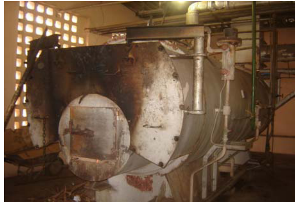
Fig. 1 Wood-fire boiler utilized for the dairy industry steam generation.
