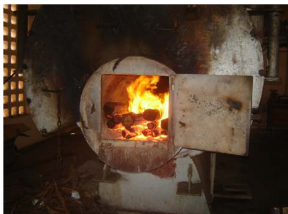
Fig. 3 Boiler in full operation during the night shift.
