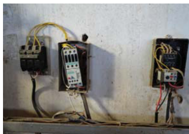
Fig. 2 – Exposed wires without adequate protection against electric shocks or fire.
