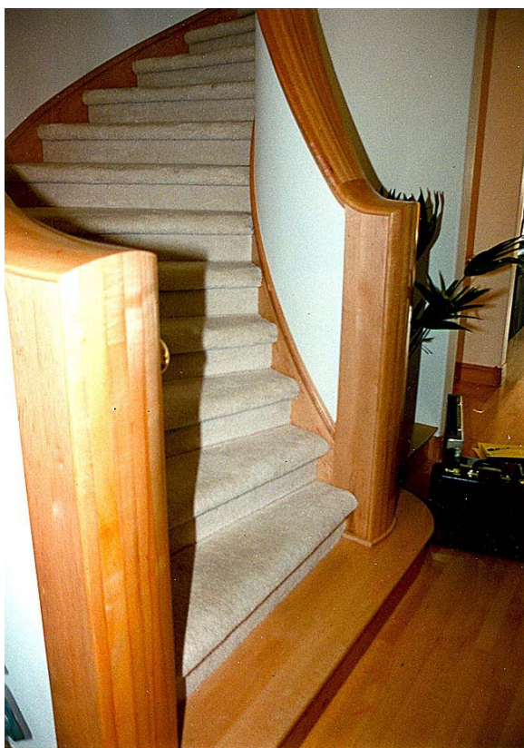
Fig. 6. In profile the bottom tread is obvious. Notice that the handrails stop short of the bottom nosing.
