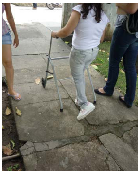
Fig.4. Photography showing a close of the sidewalk
