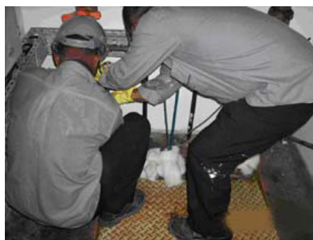
Figure 2 – Remove the check valve – Performing maintenance removal of the valve that provides that they be exposed to waste harmful to health such as bacteria. Exposing them to the ergonomic and biological risks such as back pain, tuberculosis, diarrhea
