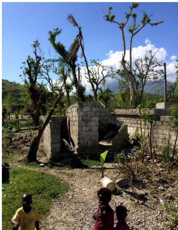
Fig. 1. Damage from Hurricane Matthew in the South.
