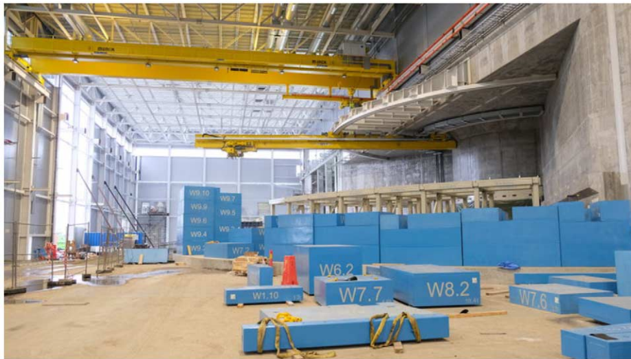
Fig. 5. Overview of the complete bunker area in the ESS D03 instrument hall.
