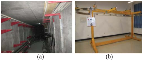
Fig. 1. (a) Underground cable tunnel; (b) the cable tunnel inspection robot system.
