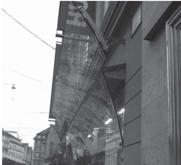
Fig. 21. Shop window with optical failures.
