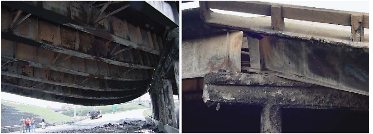
Fig. 2. From left to right, (a) underside damage to the bridge, and (b) observation of web shear buckling near the column support. Photos courtesy of the Alabama DOT.
