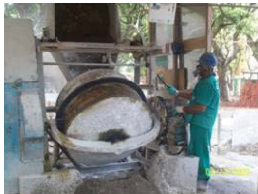
Figure 2: Mixer 2 on site "a"
