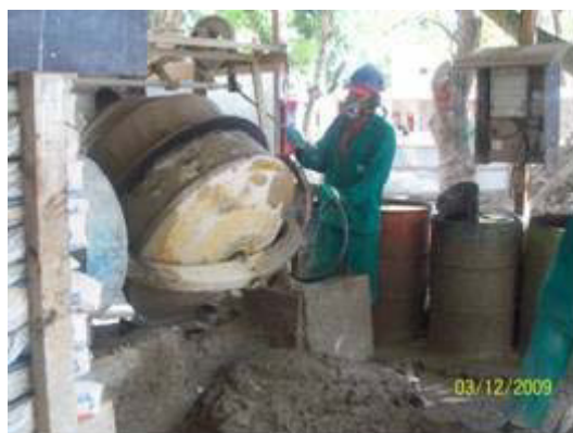
Figure 1: Mixer 1 on site "a"
